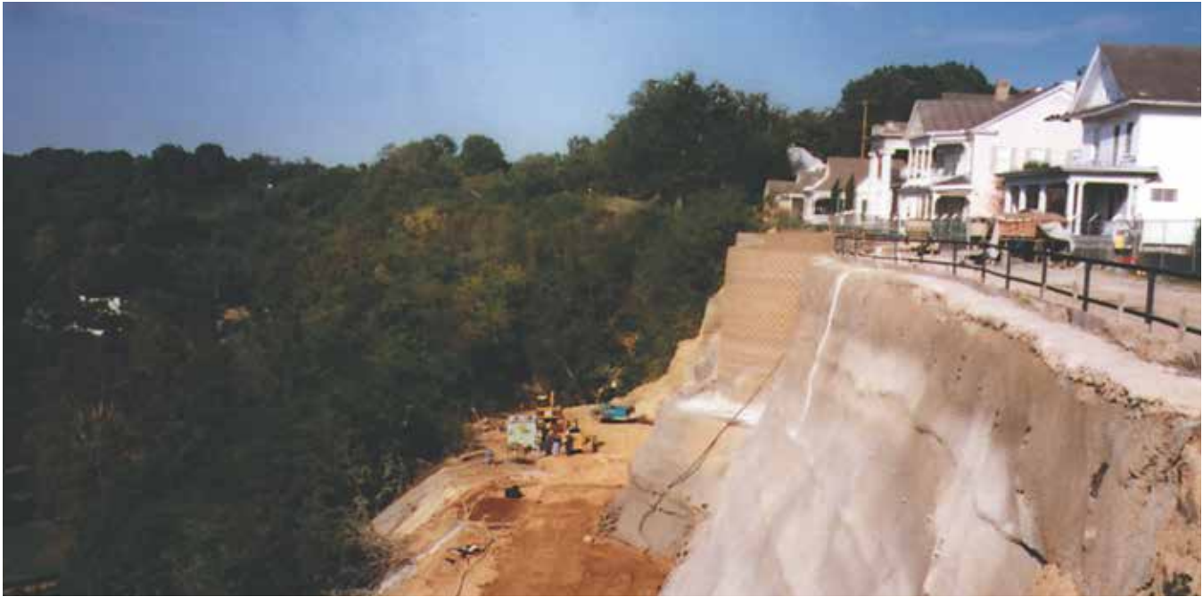
The top of the Keystone wall provides new front yards for bluff homeowners.
