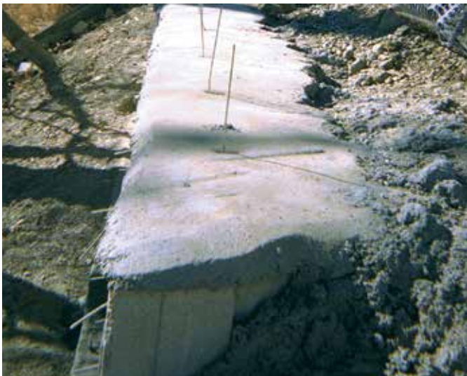
View of top of wall elevation showing grouted cap serving two purposes: (1) seal off water; (2) secure wire to units and provide clean surface for rock attachment.
